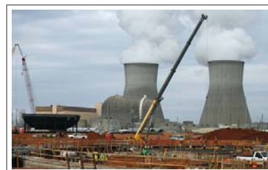
FILE -In this Dec. 11, 2012, file photo, part of the containment vessel for a new nuclear reactor at the Plant Vogtle nuclear power plant is under construction in Augusta, Ga. Some of the world's top climate scientists say wind and solar energy will not be enough to head off extreme global warming, and they are asking environmentalists to support the development of safer nuclear power as one way to cut fossil fuel pollution. (AP Photo/John Bazemore, File)
