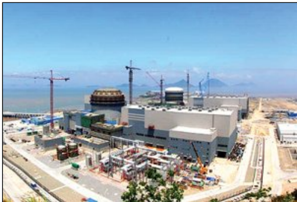
The Green River plant will be similar to this one being constructed in China.
