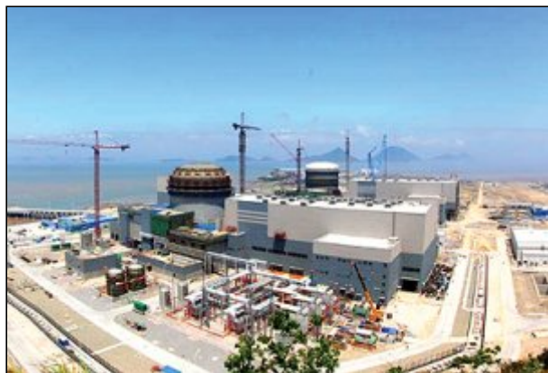
The Green River plant will be similar to this one being constructed in China.
