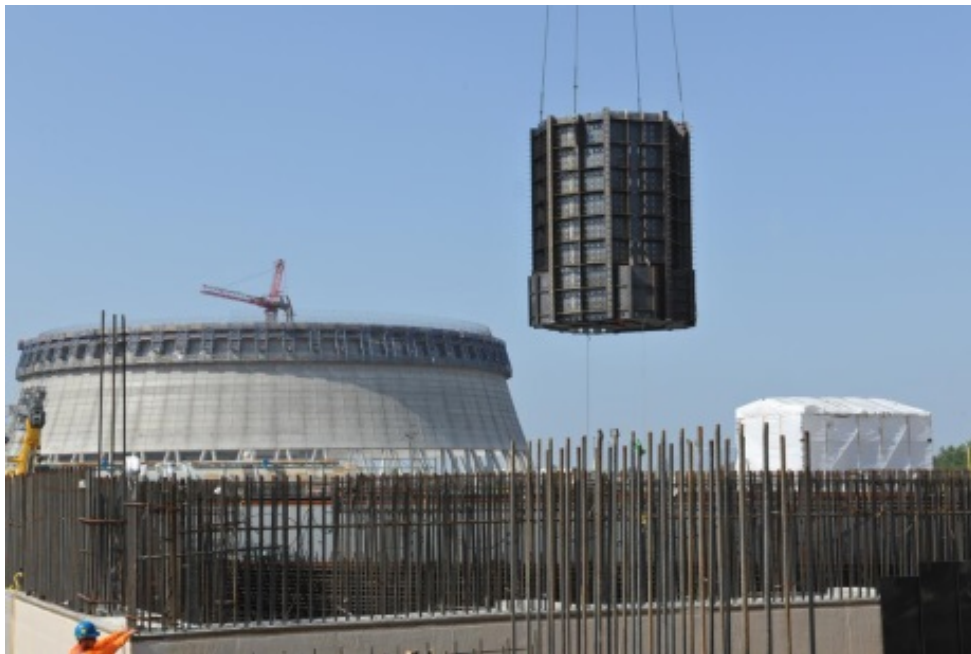
The CA04 module is lowered into place in Vogtle 4's containment vessel bottom (Image: Georgia Power)
